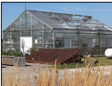
Low Park Greenhouse after the August 10, 2020 Derecho, missing most of the roof panels.
