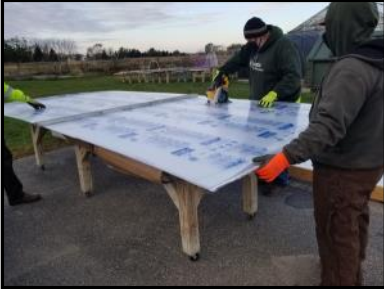
Marion Parks employees cutting greenhouse panels to fit the vent and roof.
