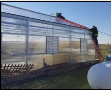
Marion Parks employees installing roof panels. The ladder is used for support as it would stress the panels to step directly on them.
