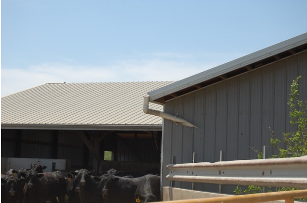
Figure 2: Use gutters to prevent clean water from entering your open lot.
