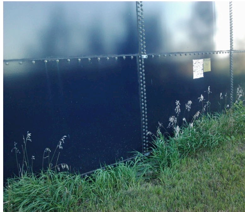
Figure 2: Maintaining area around storage structure, including mowing and tree removal, makes conducting a visual inspection easier. Photo credit: Rachel Kennedy, Iowa State University Extension and Outreach
