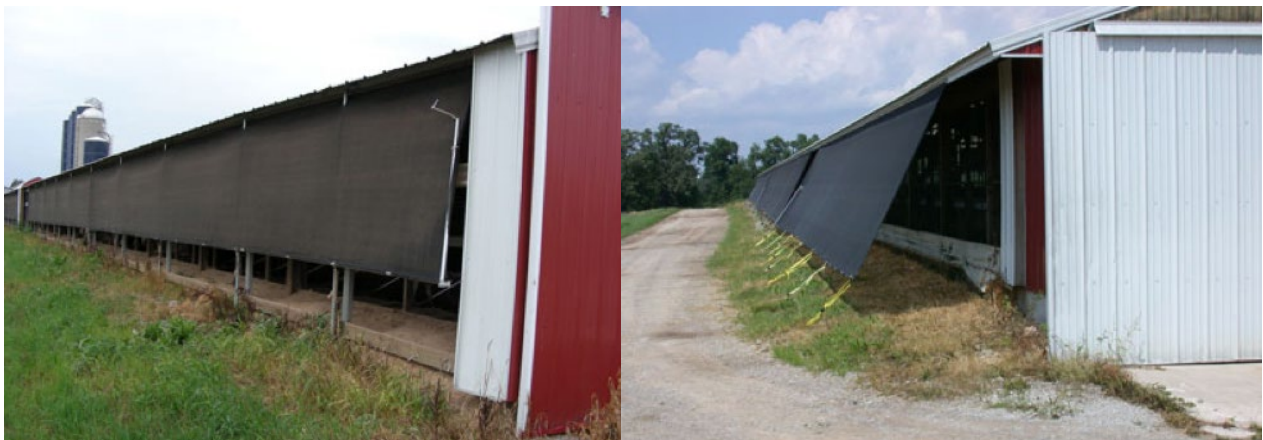
Figure 3. Shade cloth to prevent direct sunlight from penetrating into the barn. Photos courtesy the University of Wisconsin-Madison Dairyland Initiative.
