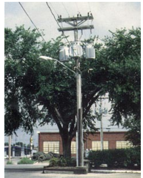
Figure 2. Grown into a power pole.
