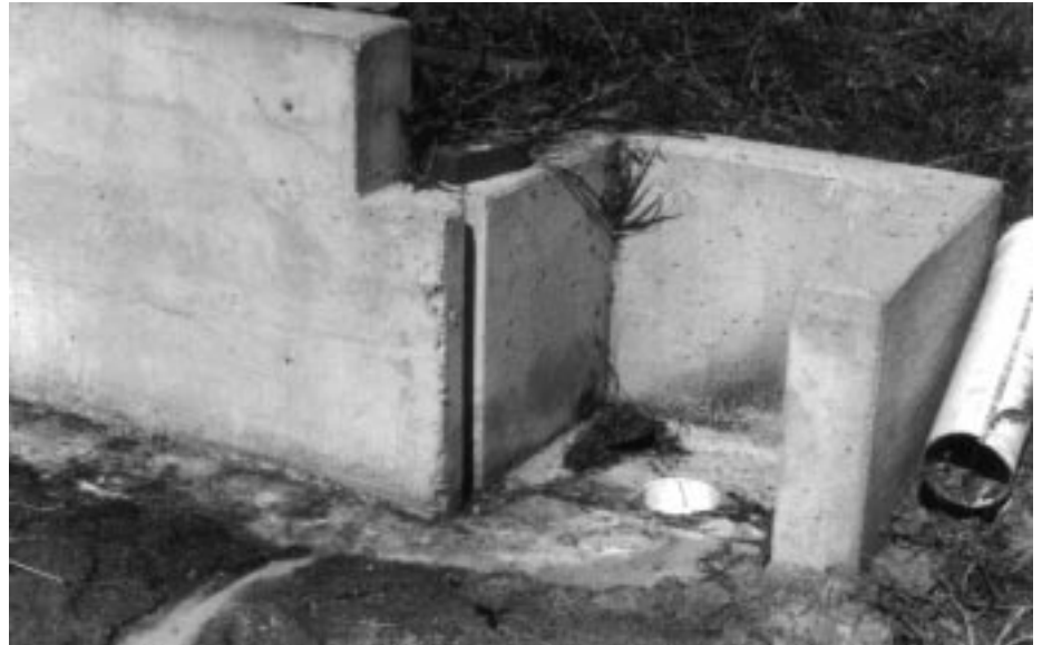
This outlet pipe carries away runoff liquids. Boards can be placed in the slots to create a porous dam.
