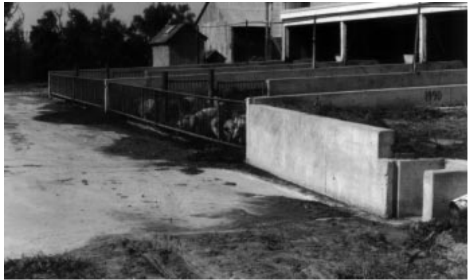
The settling apron slopes 1/10 inch per foot toward the front of this photo. The soil on the near end is graded to prevent runoff. The pipe outlet for liquids is on the far right.
