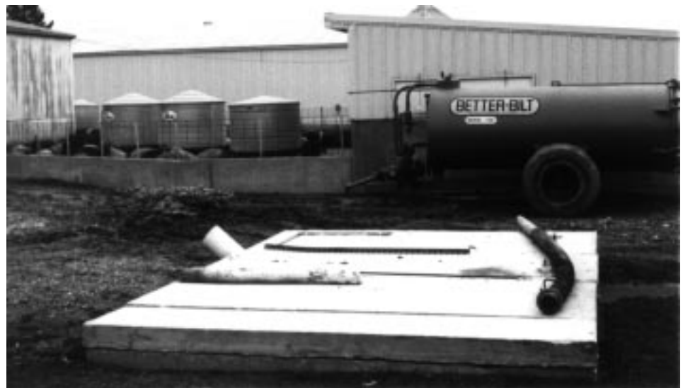
This tanker wagon is used to empty the pits. It's parked here between the west lots and the pit that serves the north lots.
