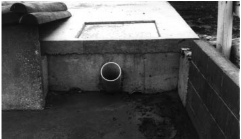
Many solids settle on the lots, rather than entering the settling tanks, as seen at the entrance to the east tank. The 8-inch inlet pipe on the right is nearly submerged.
