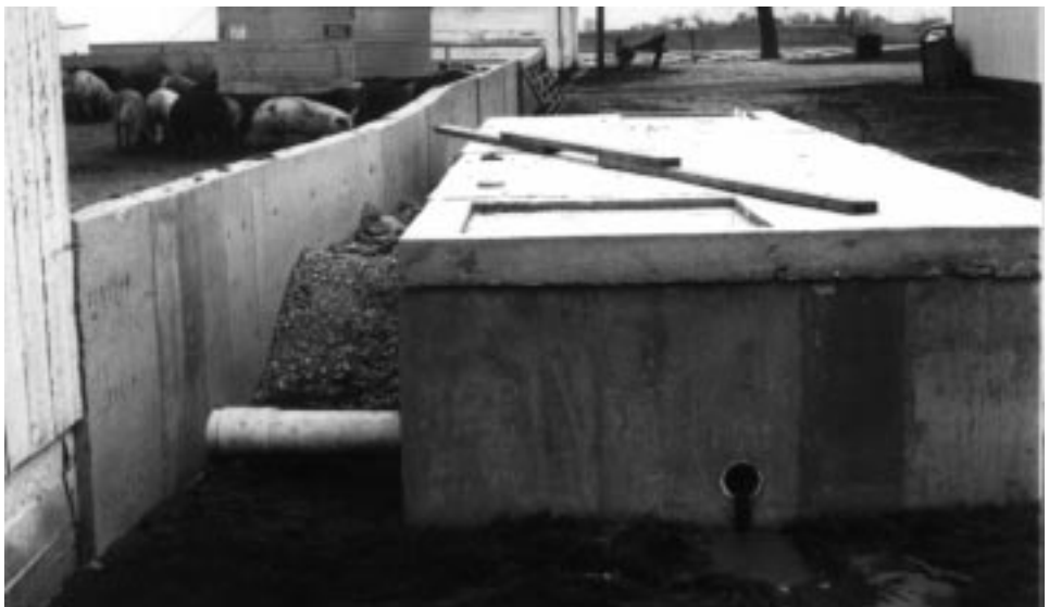
Both the inlet pipe from the lots and the outlet pipe are visible on this pit adjacent to the west lots. Note the square access opening in the tank lid.
