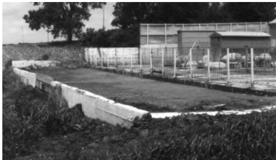
A unique feature of the system is the porous dam located at the center of the basin's side, rather than on one end.
