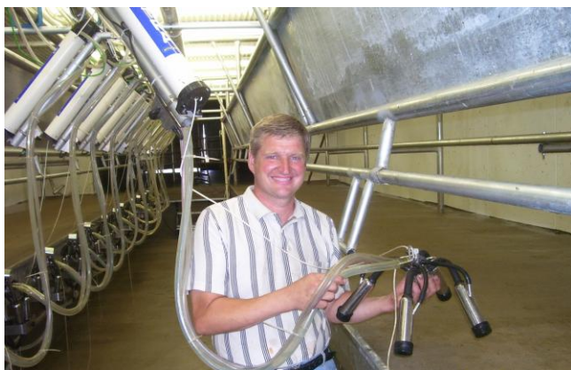
A TRANS-Iowa Swing 16 parlor designed to milk over 100 cows per hour with 2 people in the pit built for $2,350 per stall including the parlor equipment.
