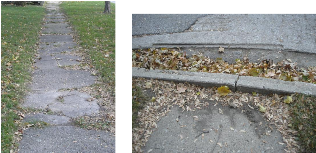
Figure 4. An extremely cracked sidewalk and a poorly kept curb.
